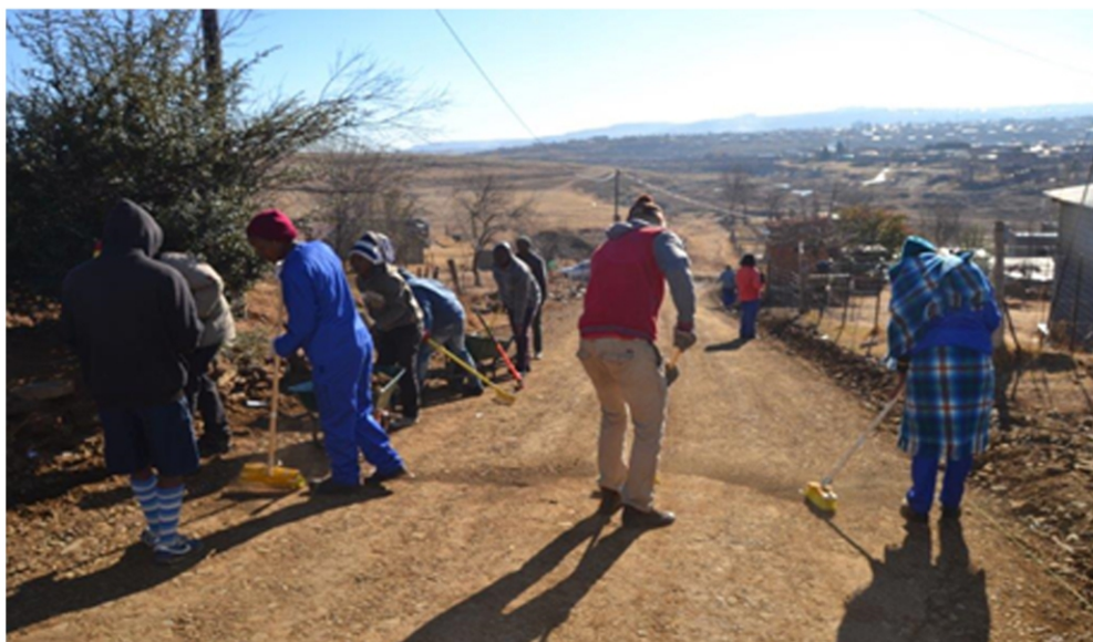
9. Preparation for the casting of the slurry by sweeping off loose material on the road surface
