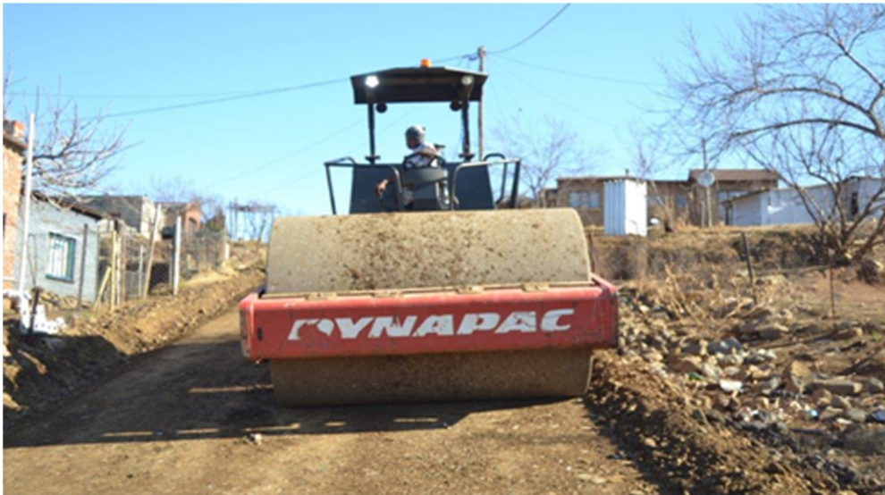
7. Screening (Preparation of the final level) through removal of loose materials by sweeping the road surface
