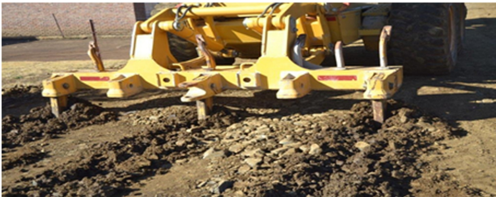
2. Ripping of the in-situ material to enable the penetration of prepared slurry
